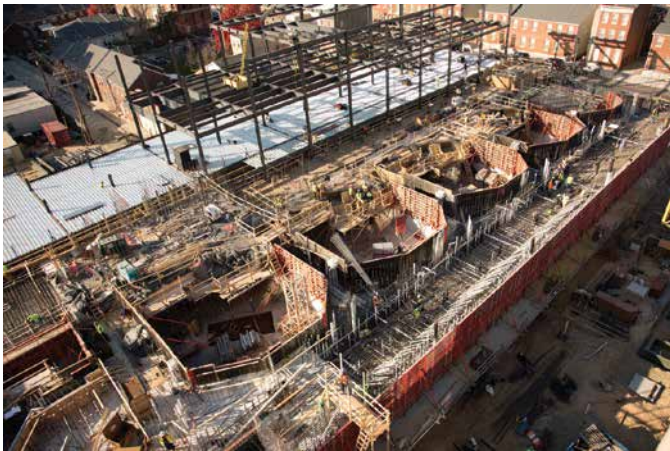
Figure 9 – Construction of gantry shielding walls at Maryland Proton Therapy Centre (source: http://www.schusterconstruction.com/projects/maryland_proton_treatment_center.html ).
